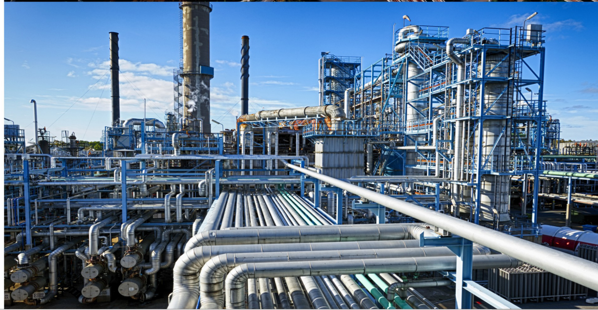
化工厂 chemical plant
